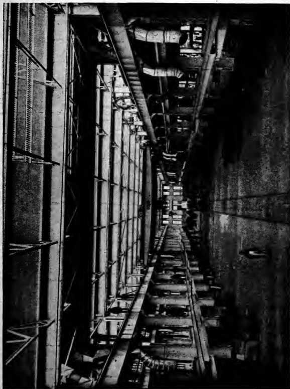
Typical Layout of Piping Showing Main Ducts and Branch Outlets, as used with Fan System Heating Apparatus in a Machine Shop
